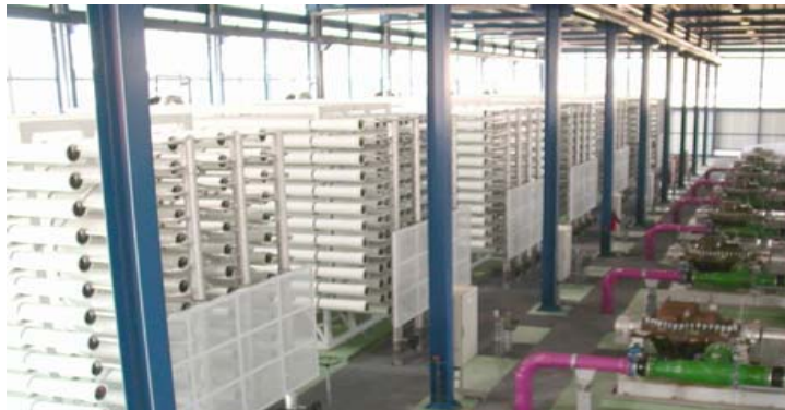
Sea Water Reverse Osmosis Plant
